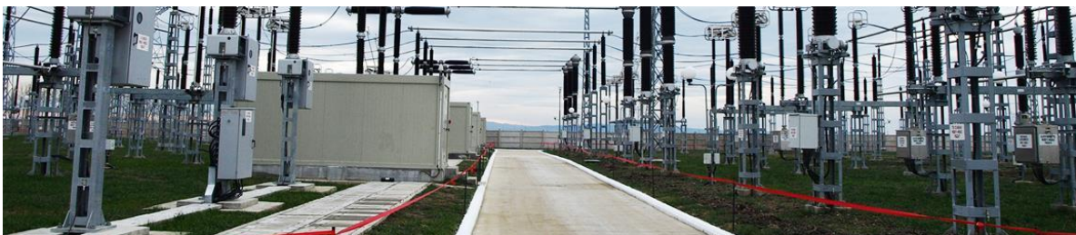
Figure 3. Fintinele Power Station.
